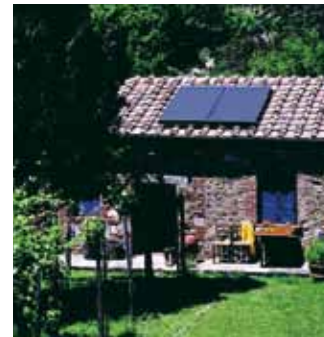
Vitosol 200-FM com ThermProtect instalado numa moradia unifamiliar.
